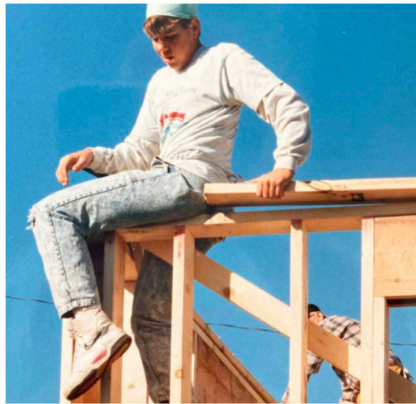
A St. Paul's youth shows no fear of heights while helping build a Habitat house.
